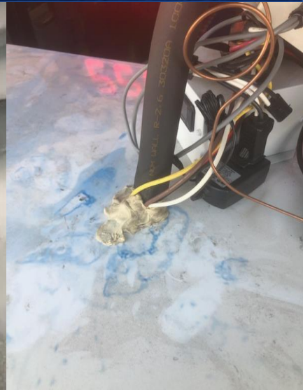
Auto-Defrost – “Snake Cable through evaporator”
